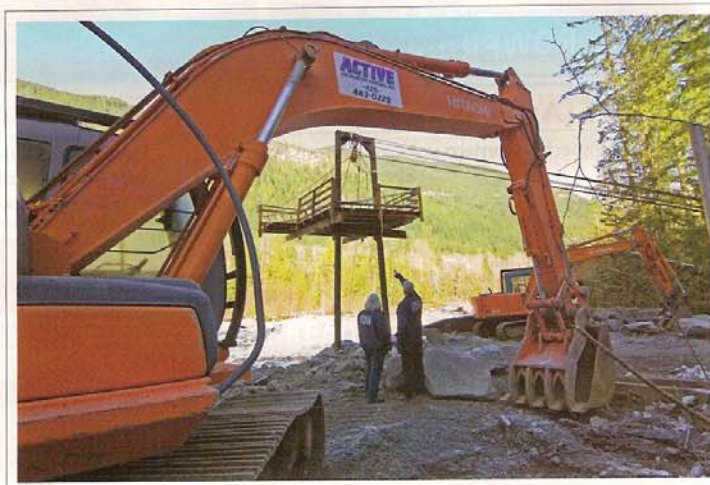
Index, WA, 1/27/07 - Two FEMA workers point to where the stairs used to be attached to this sky tram before flood waters washed the stairs and part of the landing away. This is the only access to a resident's house across the river. FEMA helped replace the stairs and landing with its Individuals and Households Program. Marvin Nauman/FEMA photo
